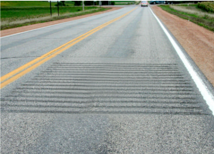
Figure 1-1: In-lane rumble strips, full width
