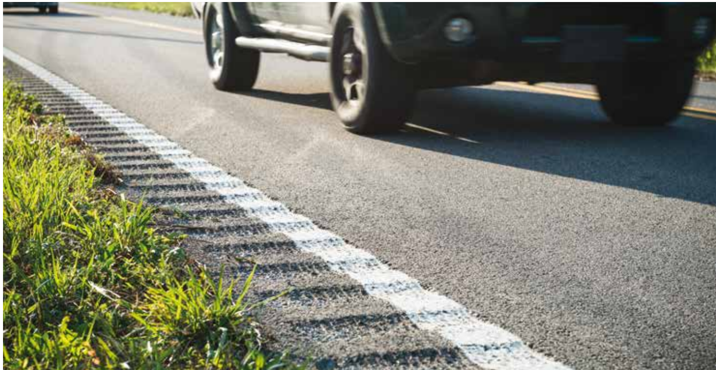
Figure 6. Photo. Pattern of depressions cut into pavement surface creates sound and vibration to alert drivers who are drifting out of the travel lane. ©Joel Carillet/iStock.
